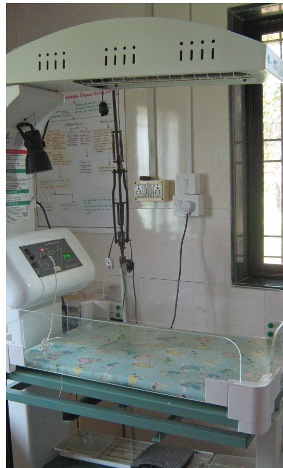
A functional SNCU equipment powered by SHPV system
