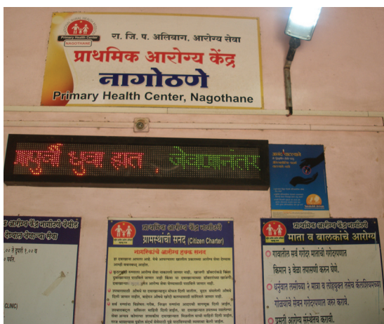
Solar powered light and electronic message board at Out Patient Department in PHC, Nagothane
