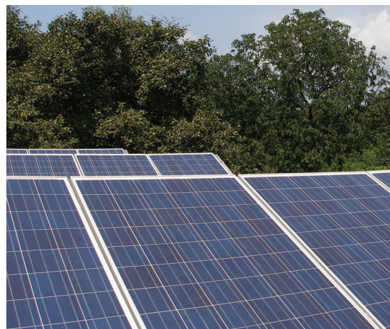
Solar panels on roof of PHC, Nagothane
